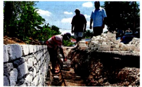
Gunarajah (right) inspecting the construction of wider drains in Jalan Tan Sri Manickavasagam 9, Taman Menara Maju in Klang.
